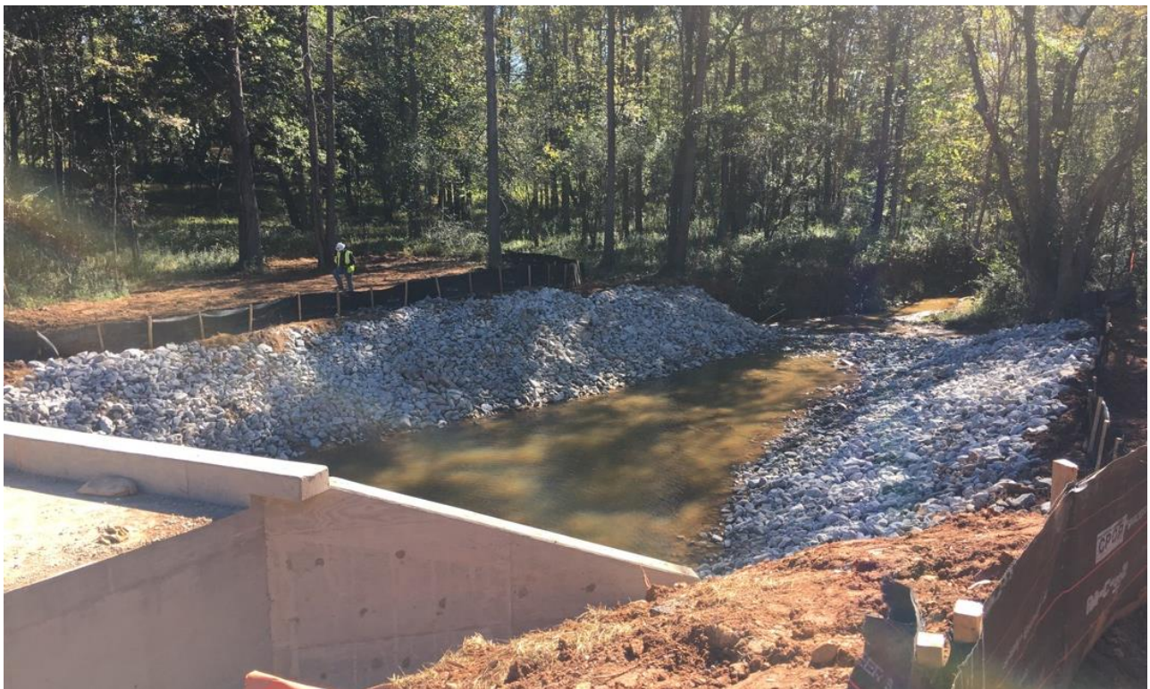
Photo 2: South of culvert: Filter fabric and rock is complete on both sides of the creek.
