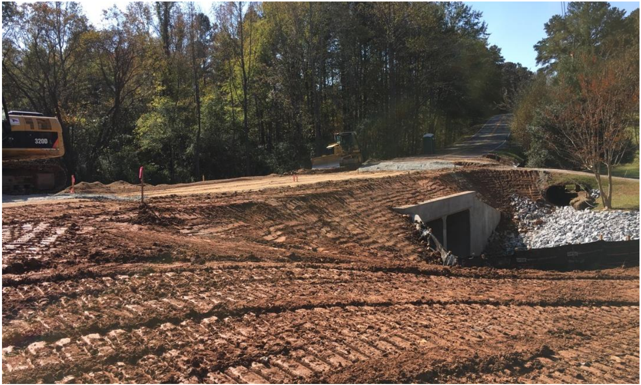
Photo 1: Backfill, compaction and grading continue at the work site, in preparation for paving. (11/02/17)
