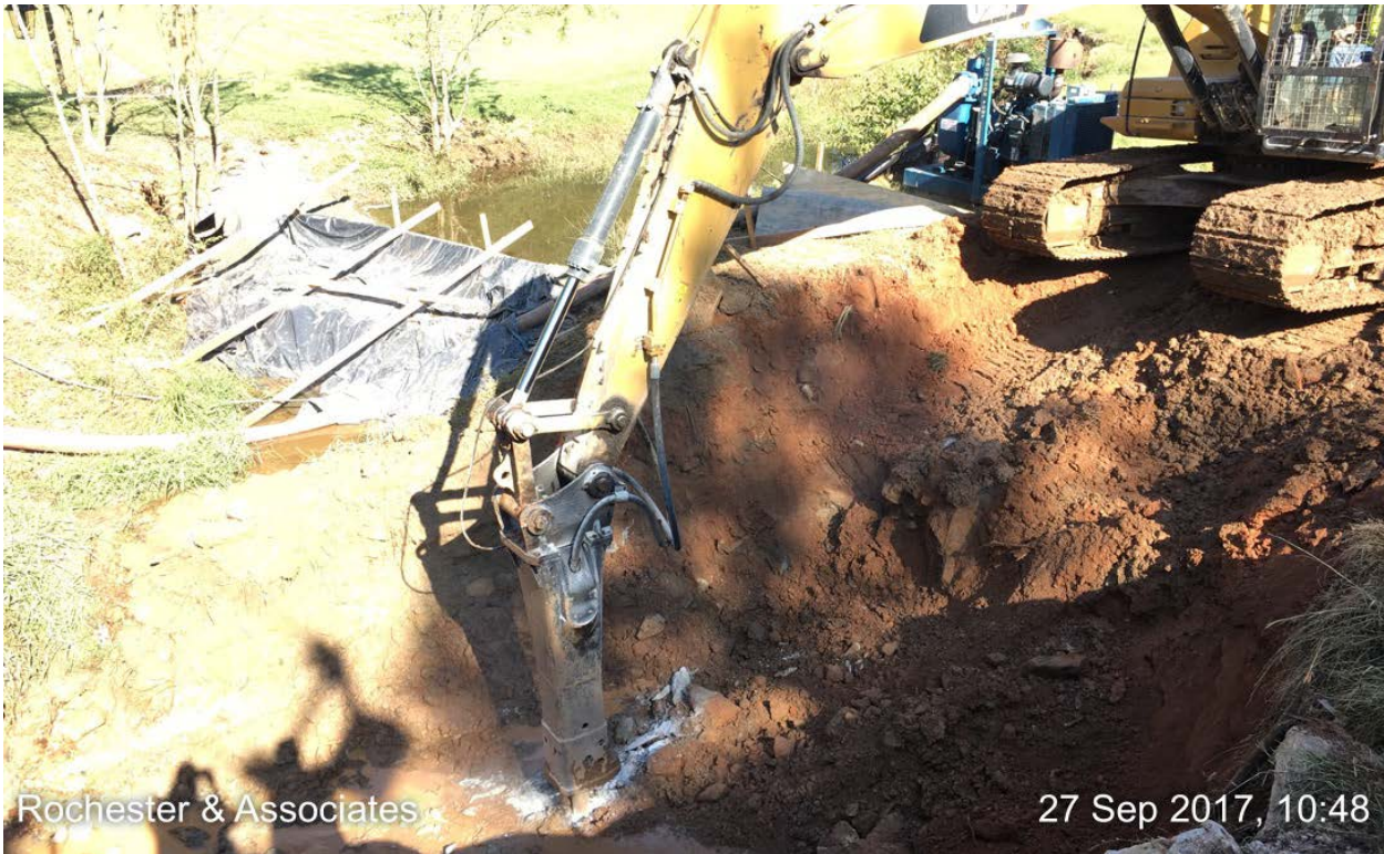
Photo 1: Excavation in the creek bed on the north side of the culvert.
