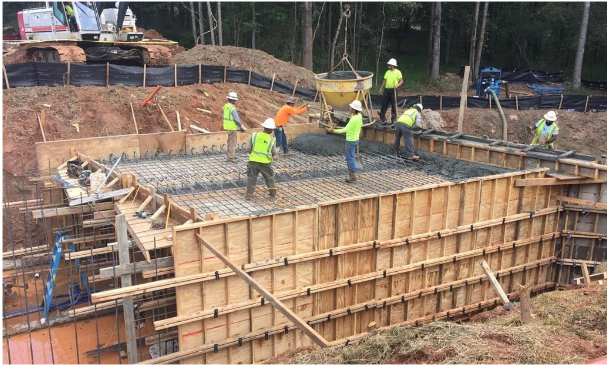
Photo 1: Concrete is being poured for the first half of the culvert walls, wings, and top.
