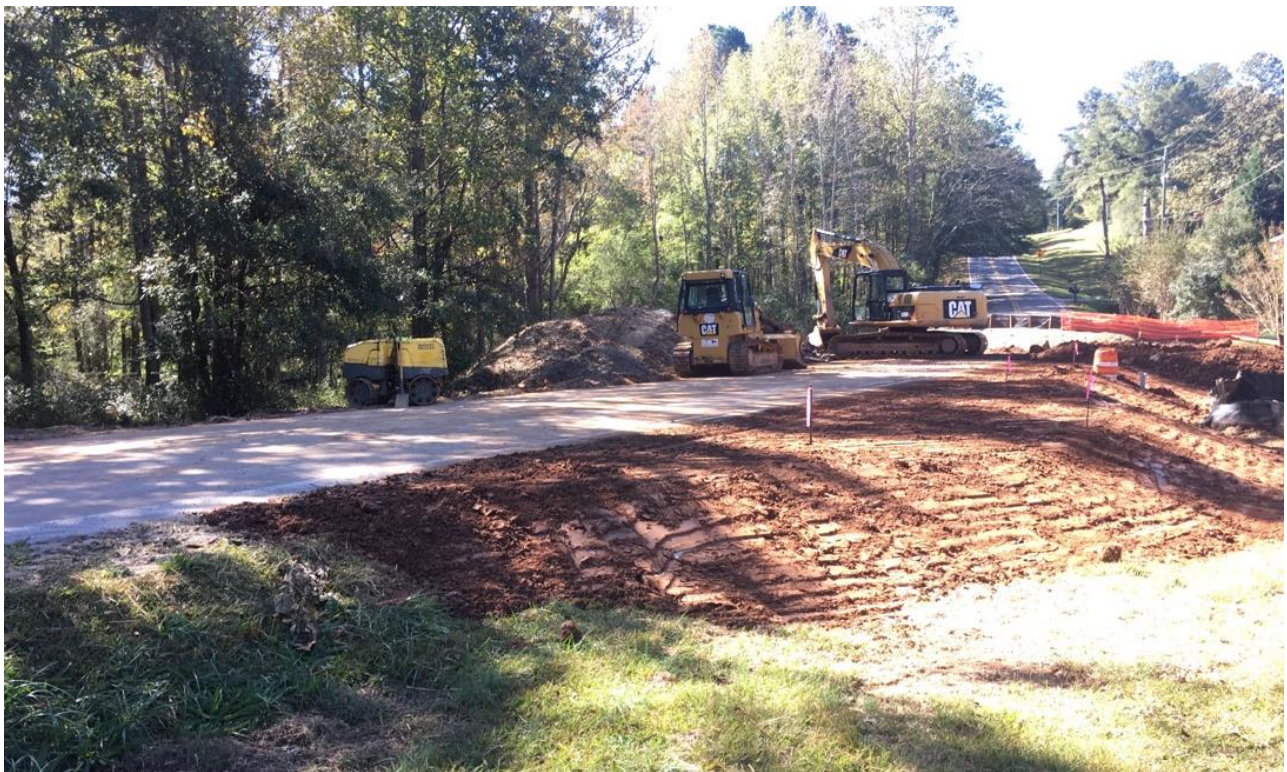
Photo 2: The shoulder area has been graded and prepped for the guardrail pad. (10/26/2017)
