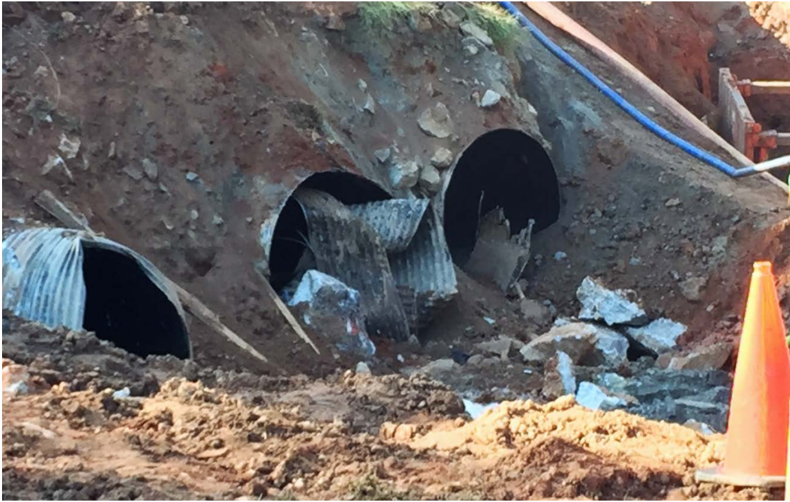
Photo 1: Tar Creek has been diverted. The ends of the corrugated metal pipes were exposed and removed on the north side of Lee's Mill Road.
