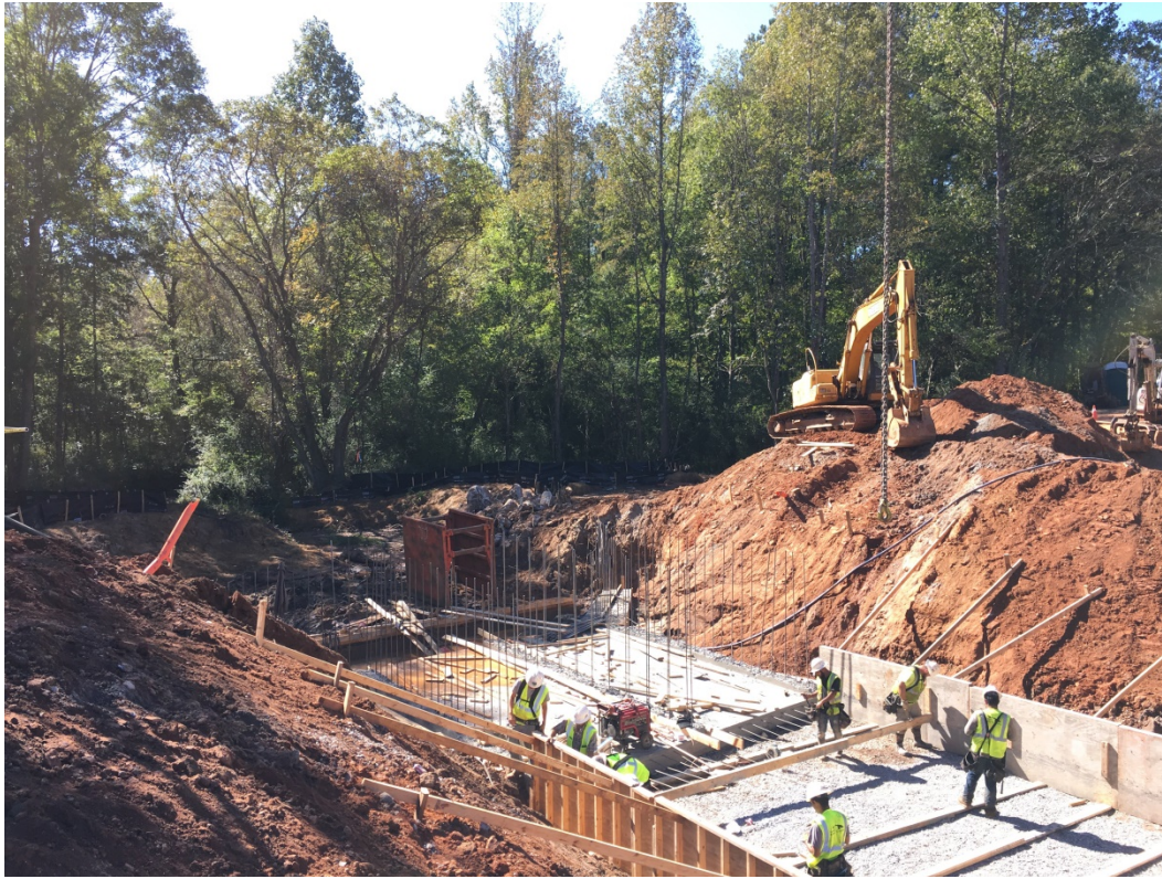
Photo 1: The bottom plate and wingwall footer construction is complete for first half of new culvert. Concrete forms and rebar are being placed for second half of culvert.
