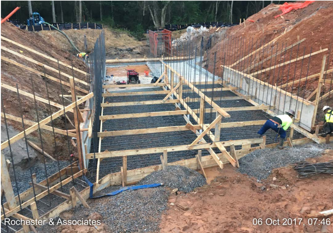
Photo 1: Concrete forms and rebar are placed for construction of final section bottom plate and wingwall footers.
