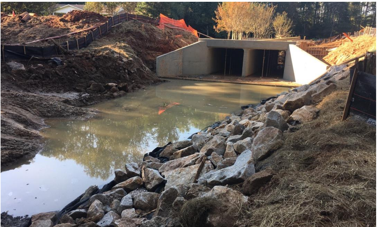
Photo 2: South of culvert: Filter fabric and rock have been placed on creek grading.
