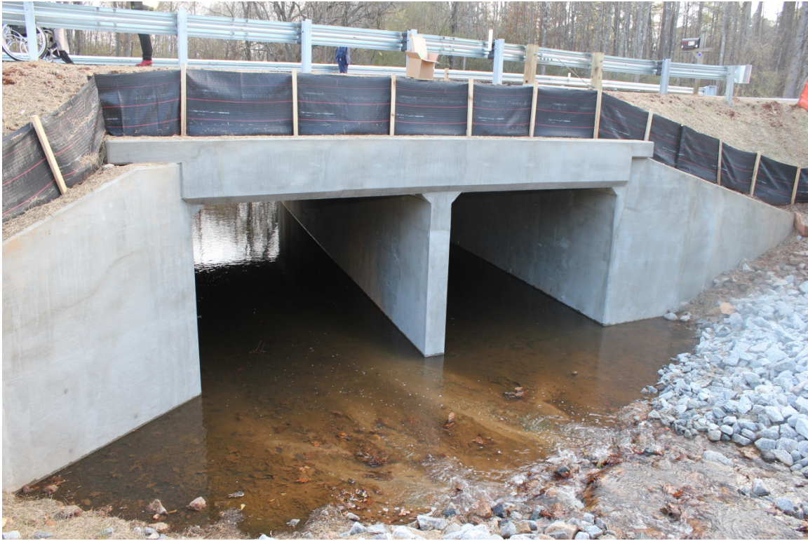
Photo 1: Culvert is open to flowing water. Roadway has been reopened to traffic. (12/14/2017 – Road was reopened on 11/16/2017)
