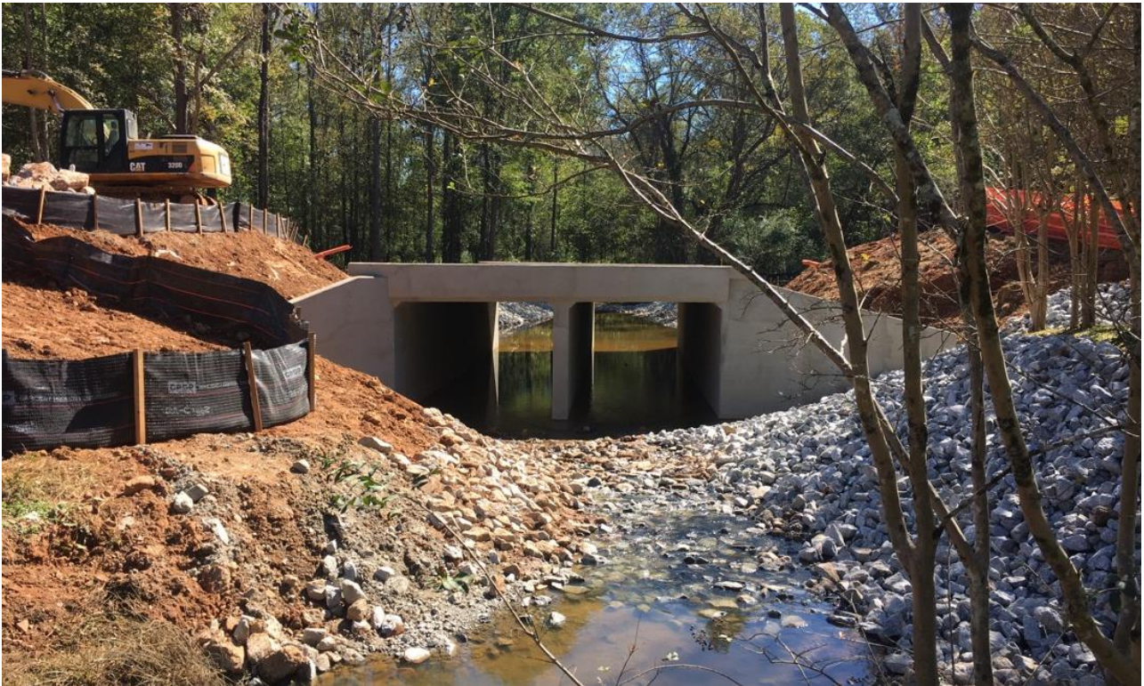
Photo 1: North of culvert: Silt fence has been reinstalled around the excavated soil along the northwest bank of the creek (left side of culvert). (10/20/17)
