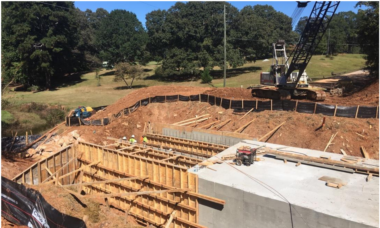
Photo 1: Concrete forms for the 2 nd half of the culvert are being installed. The first half of the culvert is complete.
