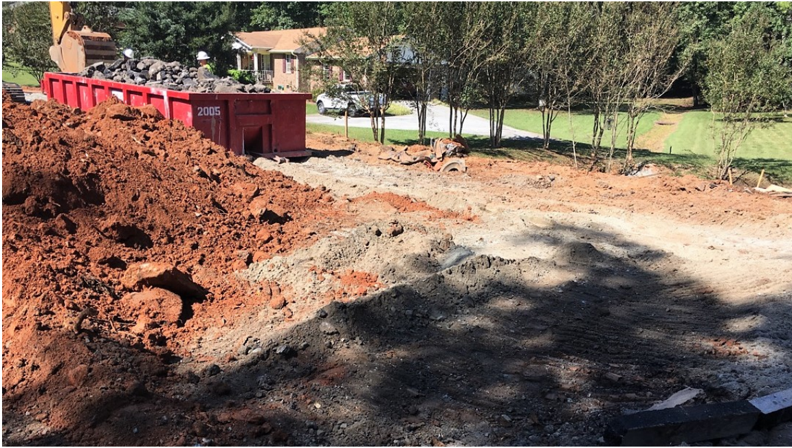
Photo 1: The asphalt is being cut and removed from the roadway, to allow culvert access.
